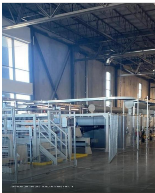
Figure 26: ZenGUARD Coating Line at Guelph Manufacturing Facility (Source: Company Documents)
